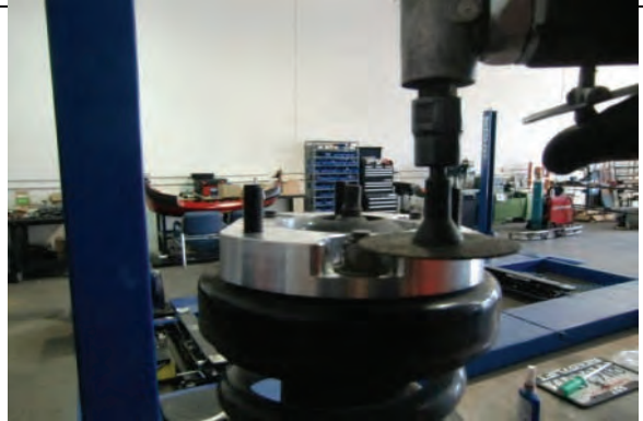
Use cutoff wheel or grinder to trim OE studs flush with spacer
